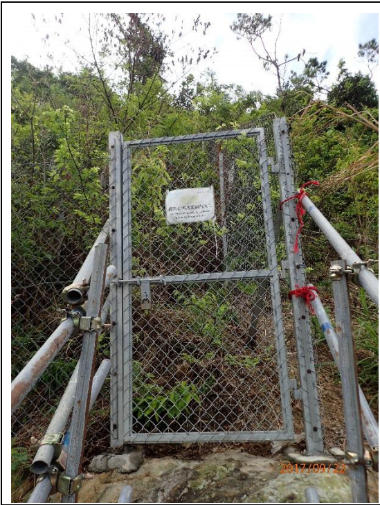
Photo 3 – Current situation of fencing and warning sign
